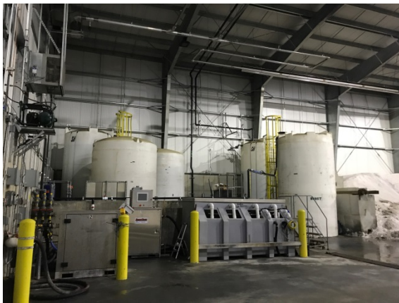
Anchorage ADOT Brine storage tank
